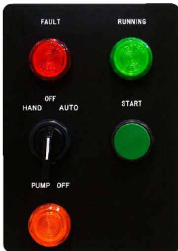
A panel located on the front of each SALT unit provides immediate access to basic control capabilities and status information
